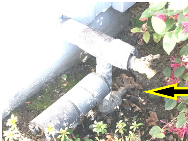
HOUSEHOLD MAIN WATER SHUT OFF VALVE
